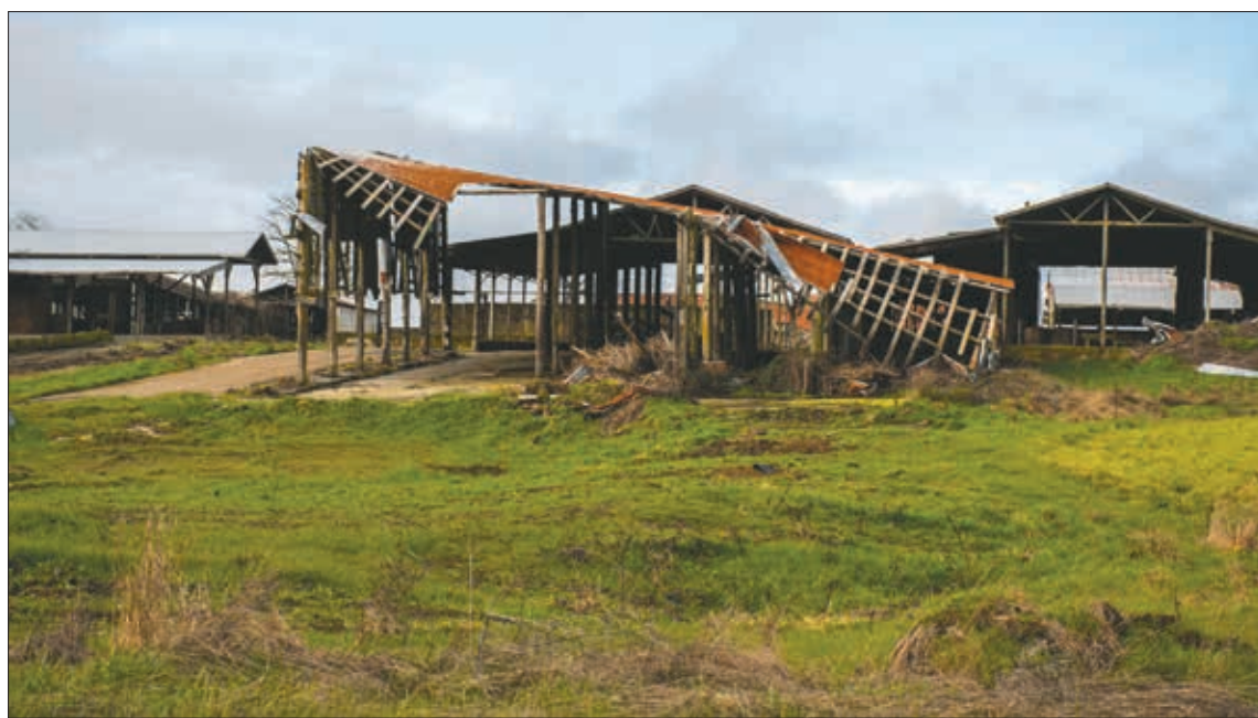
Roofs of dilapidated structures are seen off Mickelsen Parkway in Winlock during a tour of the property Tuesday morning.
