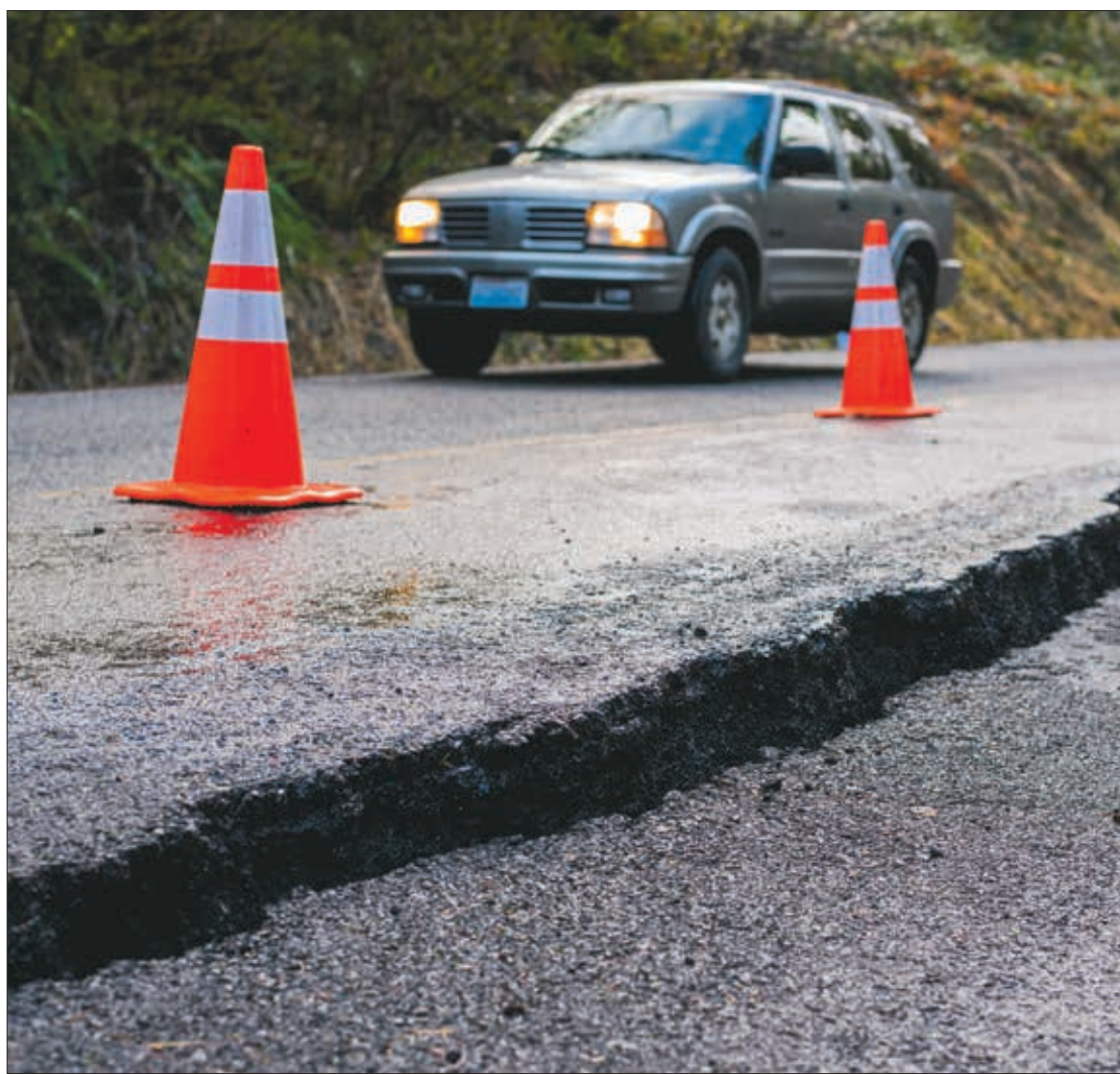
A vehicle drives past traffic cones warning drivers of a hazard along Little Hanaford Road Thursday in Centralia.
