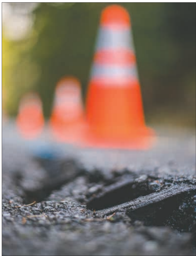
New pavement stretches across a split in Little Hanaford Road Thursday in Centralia.
