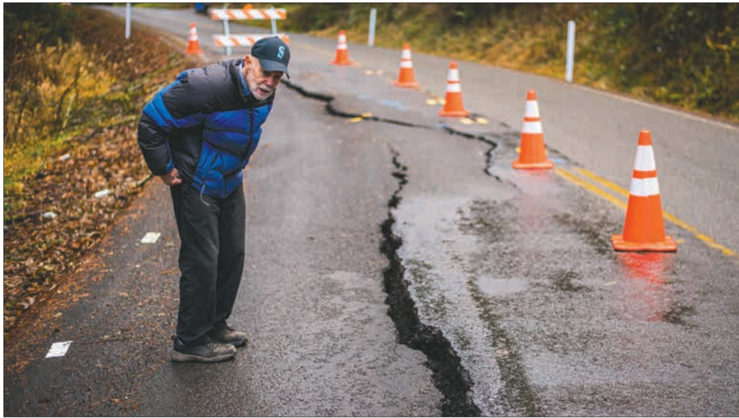
Erik Dahl, 84, looks down at a crack which continues to form in the 2100 block of Little Hanaford Road Thursday in Centralia.
