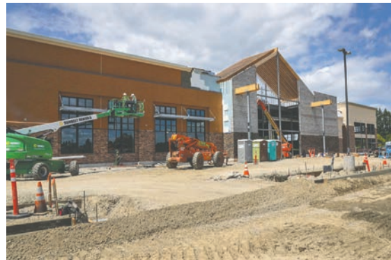
Construction crews work on the site of the future Rosauers grocery store in Ridgefield July 18.
