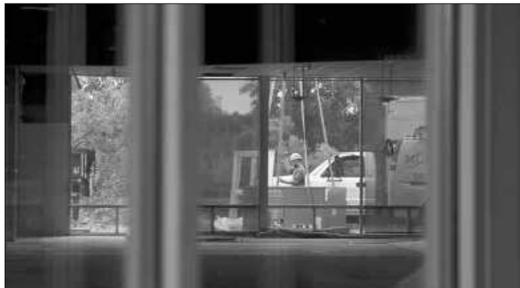
A construction worker gives the “thumbs up” to the crane operator to lift a new air conditioning unit on top of a vacant shop on Wednesday at the Centralia Outlets on High Street.
