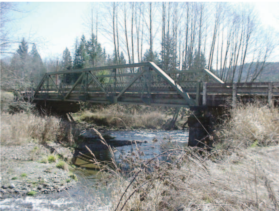
A 1930's era bridge just five miles east of Onalaska has been indefinitely closed following a routine inspection that showed significant corrosion.
