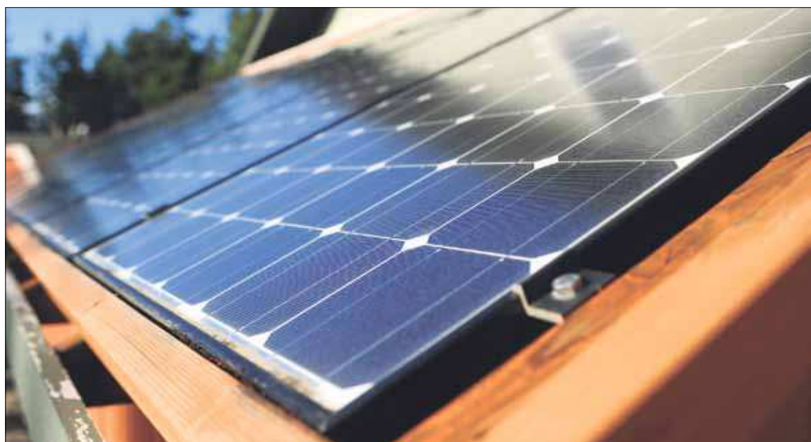
Solar panels on the side roof of Paul Munson's shed outside his home in Grand Mound are seen on Friday afternoon.
