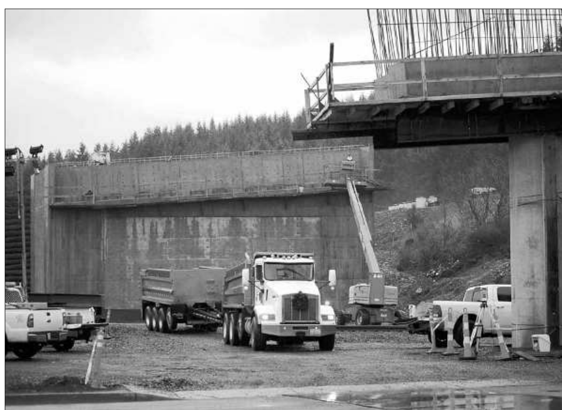
Crews finish the north abutment for a new Blakeslee Junction bridge in Centralia on Thursday afternoon.
