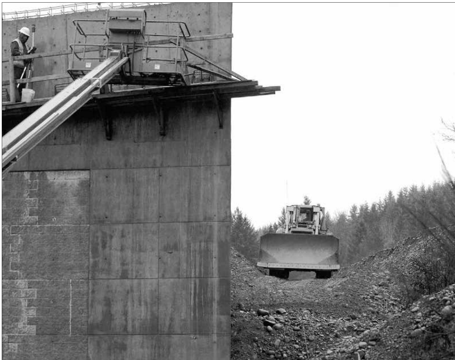
A worker surveys the north abutment of a new Blakeslee Junction bridge on Thursday afternoon.
