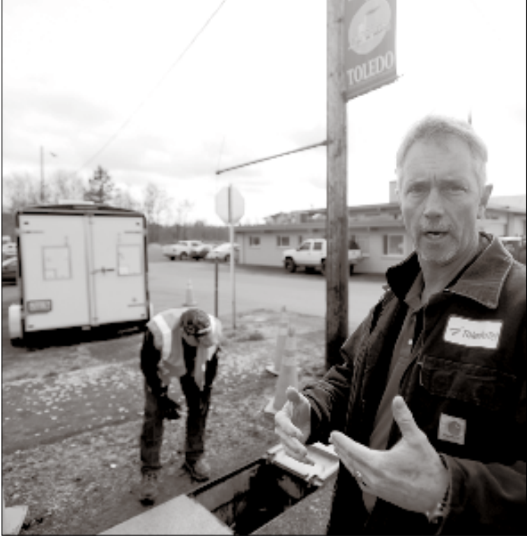
ToledoTel CEO Dale Merten explains how his company can compete with Comcast and CenturyLink as technician Greg Ockerman, left, closes up a street vault where he just finished placing a splice box near downtown Toledo on Tuesday.
