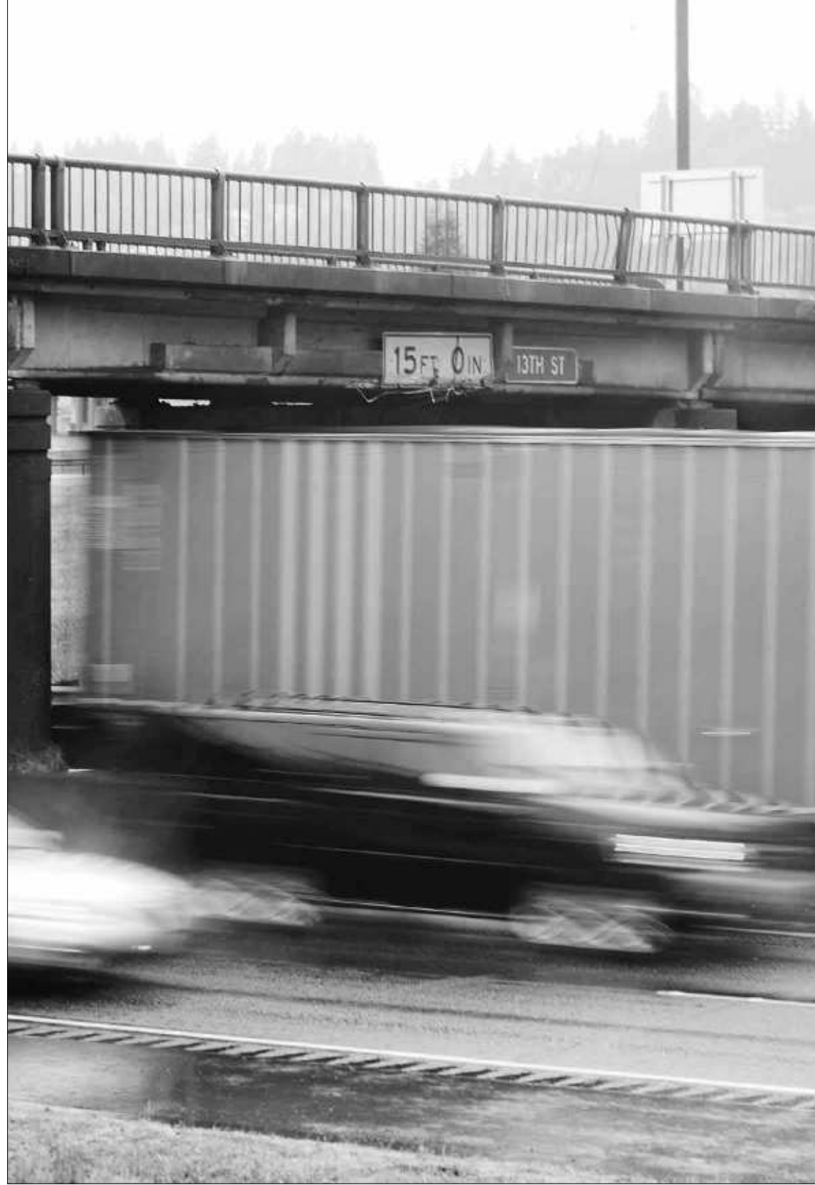
In this May 22, 2013, file photo, trucks and cars pass underneath the 13th Street overpass along Interstate 5 in Chehalis. Northbound I-5 will be closed from 10 p.m. to 5 a.m. Friday and Saturday in Chehalis while crews repair damaged girders on the 13th Street overpass, which was hit by an oversized truck last week.
