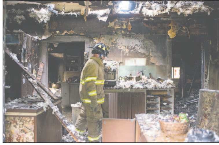
A West Thurston County Fire Authority firefighter inspects damage done by a fire at the Candy Cottage in Rochester on Thursday, May 28, 2015.
