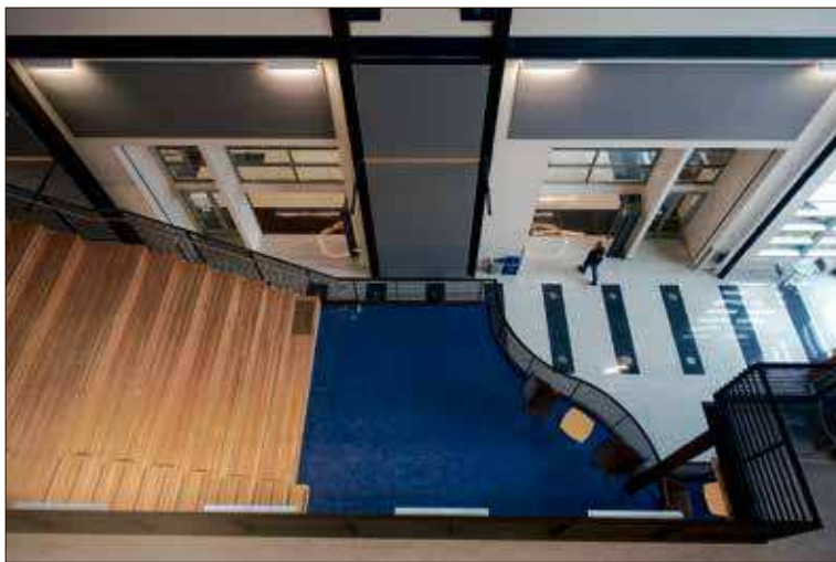
A construction worker walks into the 500-seat dining and meeting area on the first floor of the TransAlta Student Commons building on Tuesday afternoon at Centralia College.
