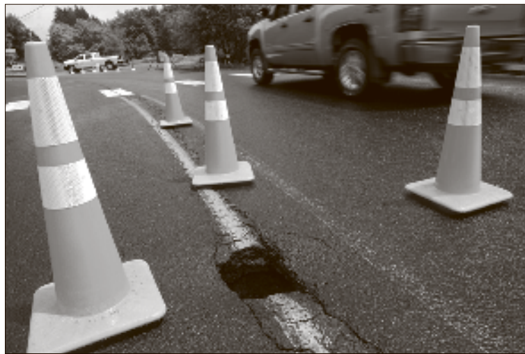
A truck drives by a small sinkhole that developed on Tuesday afternoon on state Route 505 in Winlock.
