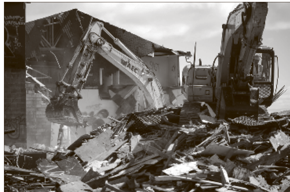
Excavators are used to tear down the former Midway Meats packing facility on Tuesday along Airport Road in Centralia. The crew from Anderson Environmental and Contracting, from Kelso, expect the demolition of the building to be finished by the end of the week.
