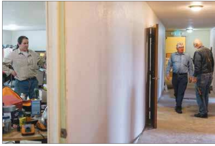
Rudy Nix, the pastor at Alder Street Baptist Church, stands in one of the larger rooms of the Centralia church as Jimmy Johnson, center, the construction coordinator for the church's rebuilding project, talks with another volunteer from North Shelby Baptist Church on Monday afternoon. A large contingent from the church came to Centralia to help rebuild Alder Street, which was heavily damaged by flooding in 2007.
