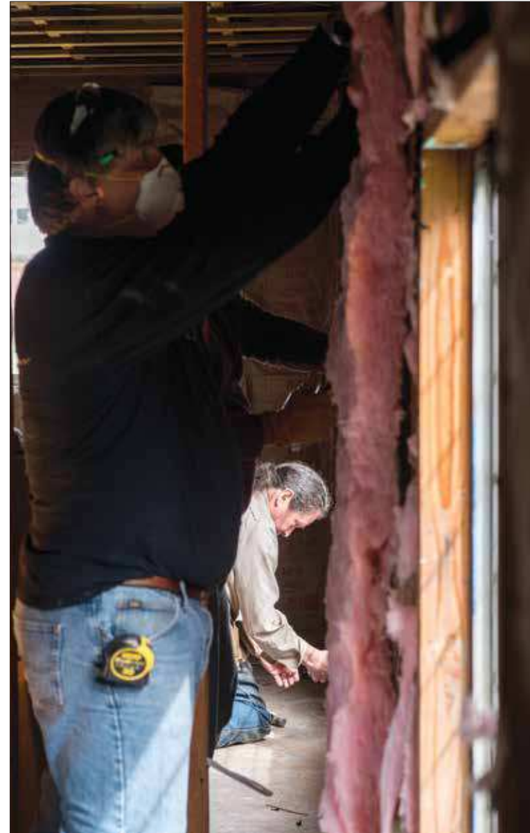
Rudy Nix, lower right, the pastor at Alder Street Baptist Church in Centralia, works alongside volunteers from the North Shelby Baptist Church on Monday afternoon. A large contingent from the church came to Centralia to help rebuild the church that was heavily damaged by flooding in 2007.
